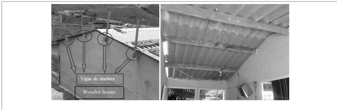
Figura 4. Vigas de madera que soportan la cubierta a dos aguas Figure 4. Wooden beams which support the gabled roof
