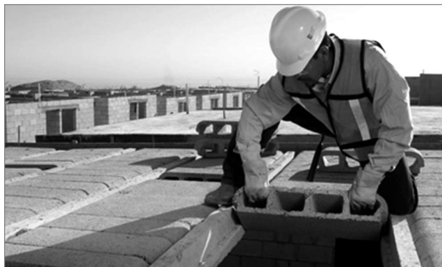
Figura 1. Sistema losa nervada de vigueta y bovedilla tradicional Figure 1. Traditional system of ceiling hoist and vault in a ribbed slab
